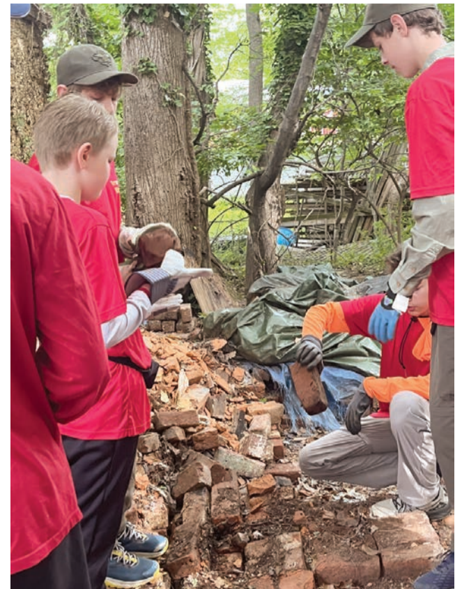
The Scouts realize the lower rows of bricks have sunk into soft soil and will have to be shoveled out.
